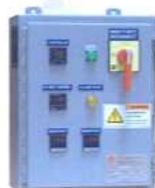
Power Control Panels
